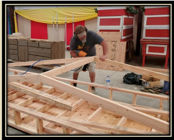
Above: John Calvert nails a rafter to the ridge board while framing the roof canopy portion of the new AVRМ Donor Wall on July 31 st . We have been fortunate to have the Small Animal Barn next to our new building as an assembly area this year, though we would have preferred to vacate for the AV Fair. John has spent many days working on the new cabinets and new building with me.
